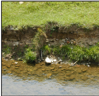
Collapse of near vertical bank after high flows have scoured the toe of the bank.
